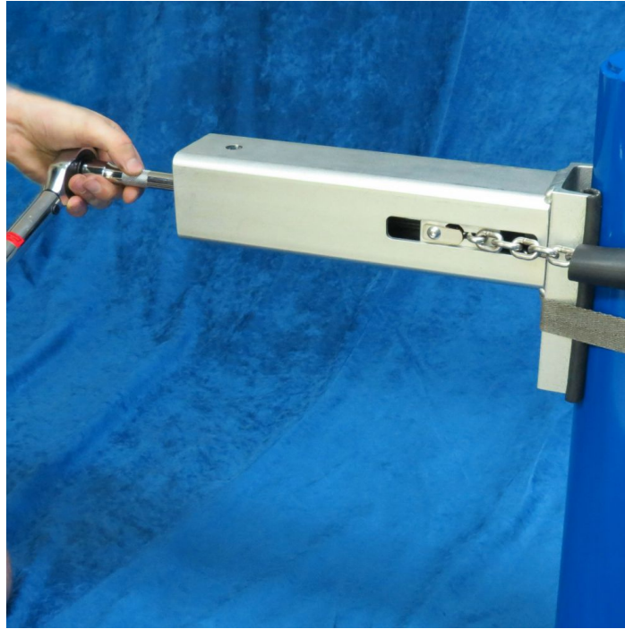
Figure 7. A torque wrench is used to apply appropriate pre-tension, and prevent bolt loosening.
